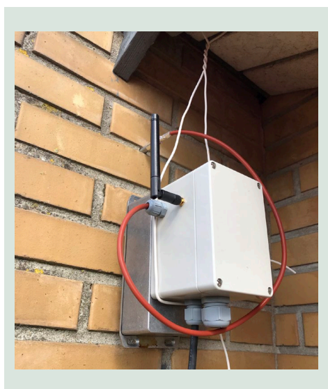
FIGURE 36. Prototype of the OptiSmoke sensor installed on a brick chimney. The red cable connects to a temperature probe. Not visible in the image is the short segment of steel pipe used as a nozzle to access the flue gas channel inside the chimney.
